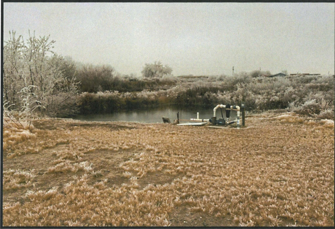
Photo 1- Near the northeast corner of the property facing north with pond and pump station in background.
