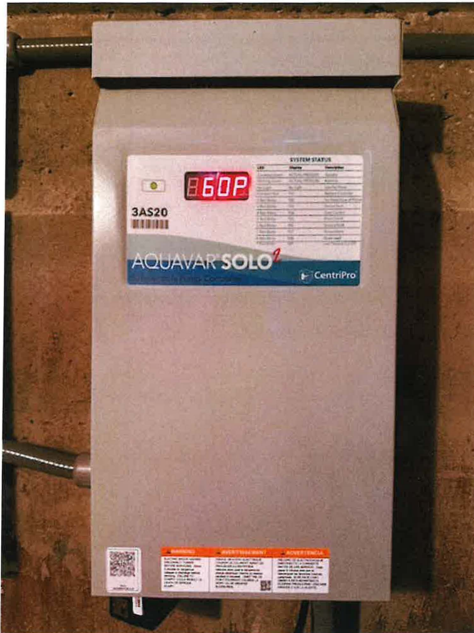
For item 2, here are some additional photos in the vault where we set up the pressure tank and filtration.
