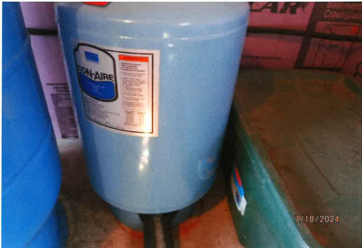
SMALL PRESSURE POT IS PART OF SURFACE WATER SYSTEM; LARGE (L/H SIDE OF IMAGE) PRESSURE TANK PART OF SEPARATE DOMESTIC WATER SYSTEM FROM GROUNDWATER WELL
