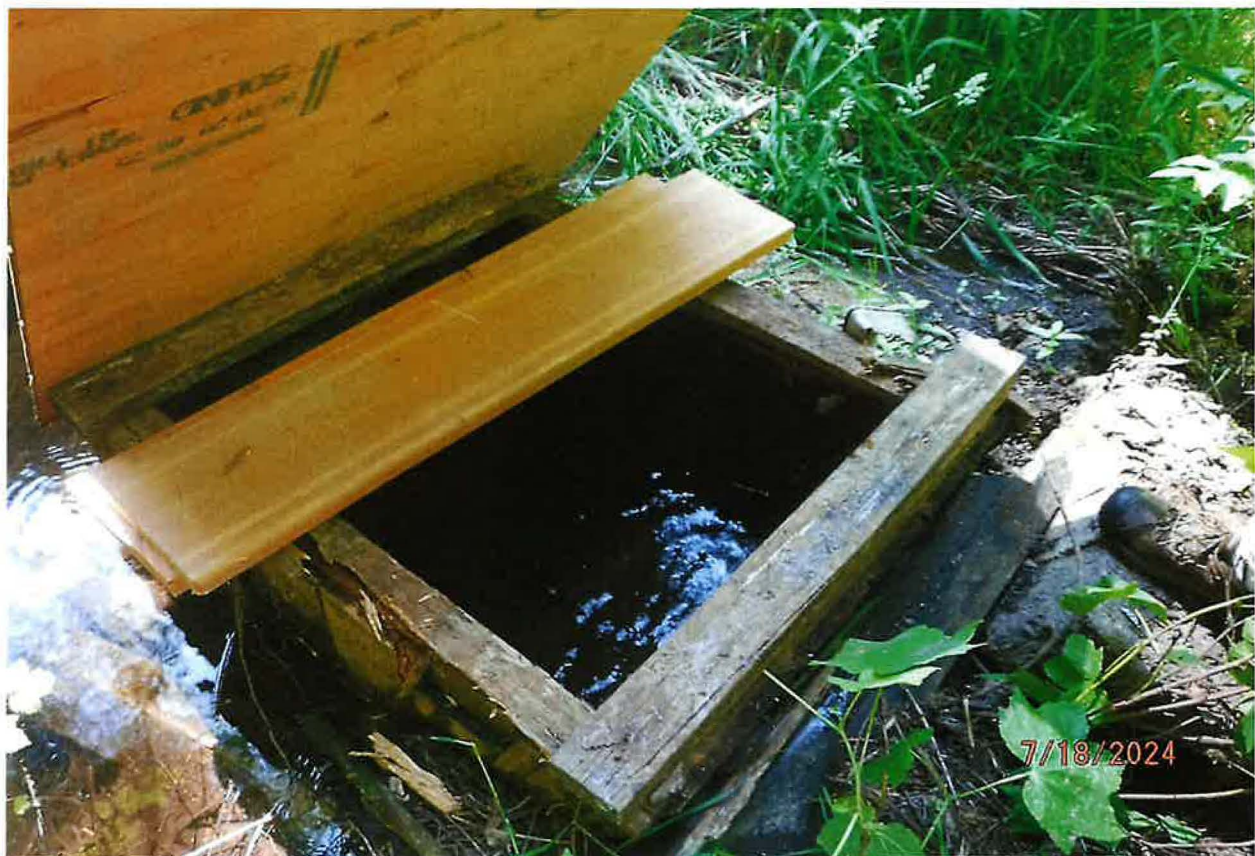
PIPE BURIED WITHIN COLLECTION BOX UNABLE TO DETERMINE PIPE DIAMETER DURING EXAM
