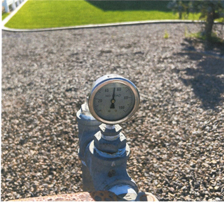
Figure 14 Close up photo of pressure gage, showing that the system is set to about 50 PSI.
