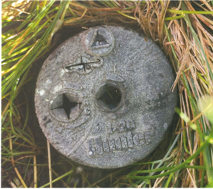
Figure 8 Hunter I-20 sprinkler head located in an irrigated lot belonging to the HOA.
