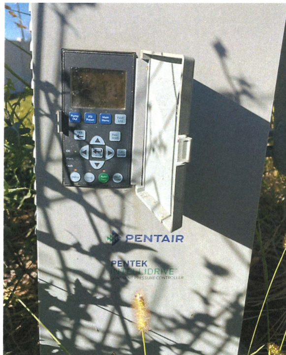
Figure 5 Pentair Pentek Intellidrive water pressure controller.
