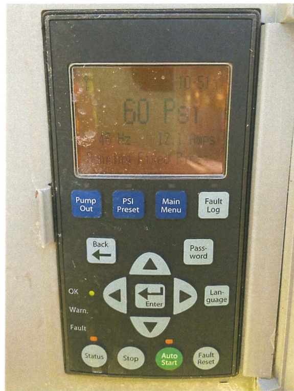
Figure 6 Pentair Intellidrive water pressure monitor screen reading 60psi.
