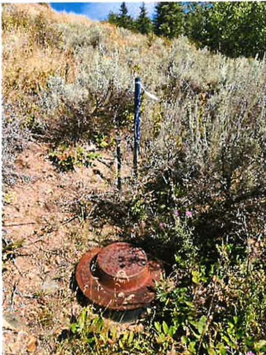
Each of the 18 buildable lots has a water connection/Shut off valve/ and water meter.
