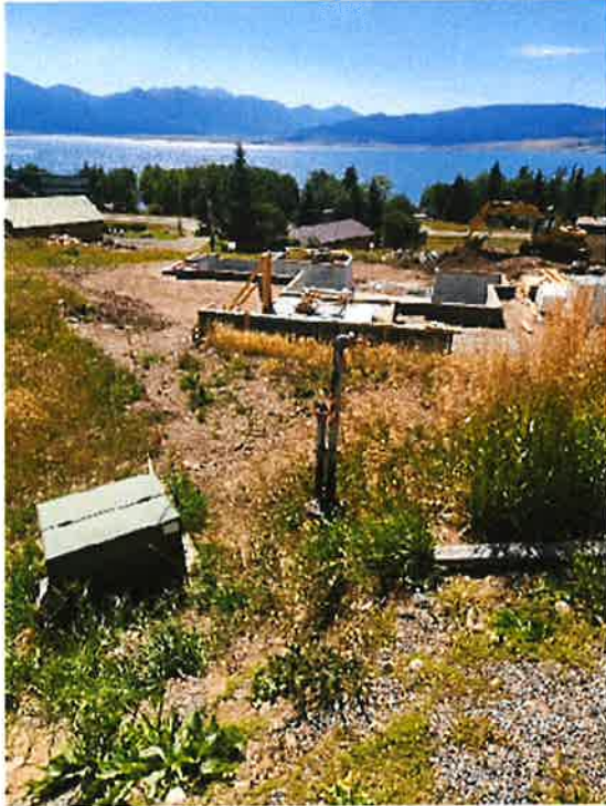
Fire suppression, 3 hook ups similar to this one located throughout subdivision
