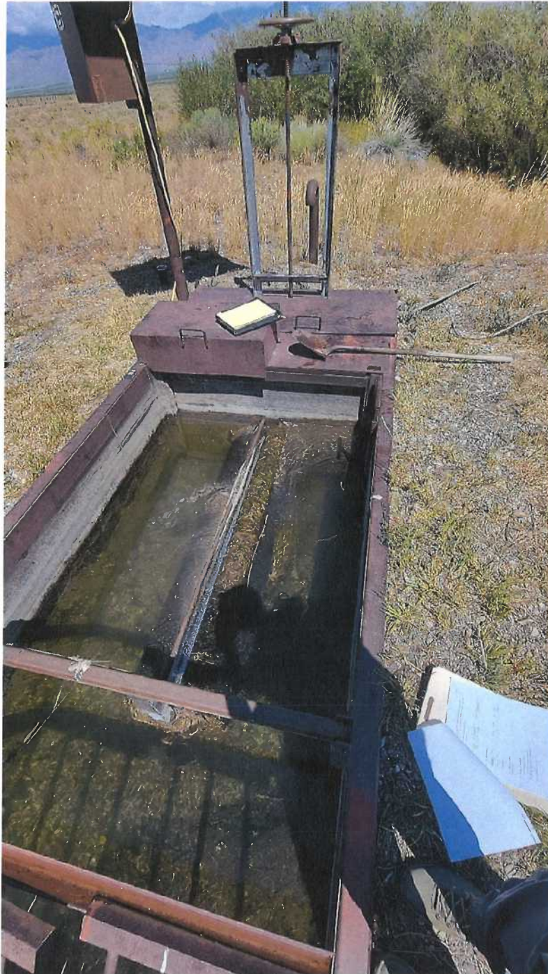
Photo 2: Fish screen/bypass. Pipeline for right 73-2A heads north towards sagebrush and willows. Fish bypass pipe heads right (east), perpendicular to the structure.
