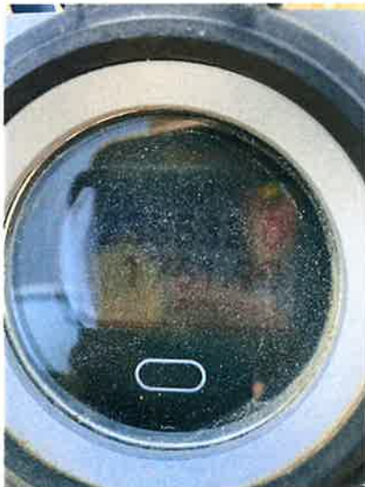
A picture of the flow meter on 7/16/24
