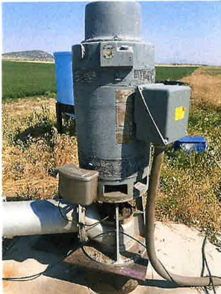
A picture of the pump and well system
