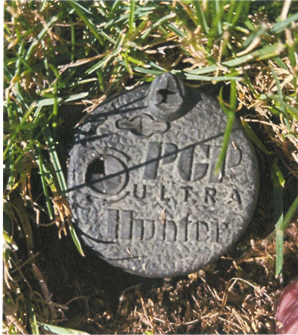
Figure 10 PGP Ultra sprinkler head located throughout the parcel.
