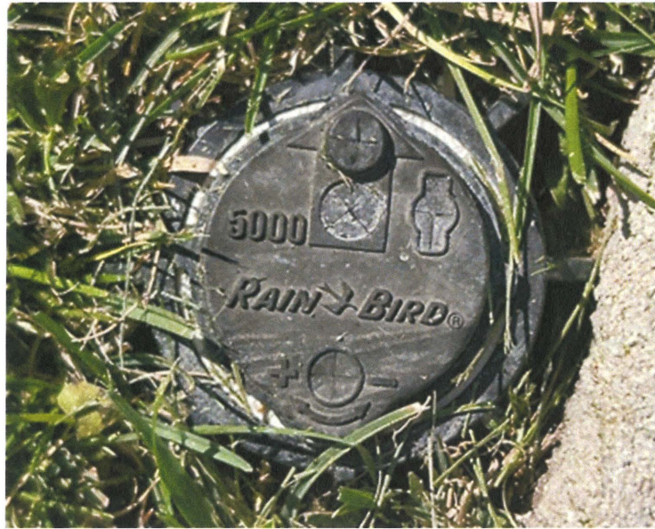
Figure 12 Rain bird 5000 sprinkler head used throughout the subdivision.
