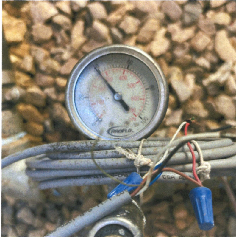
Figure 10 Pressure gage reading 40 psi for irrigation system, located at site of the well.
