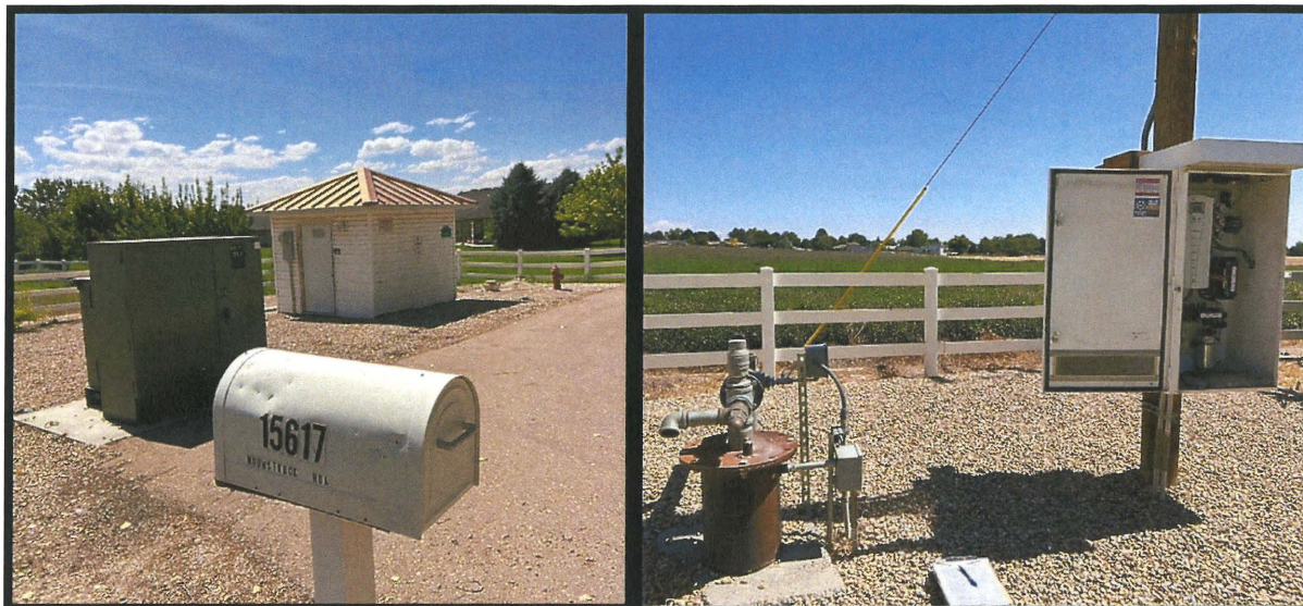
Photo1 (Left)- Well #1 Pump house, wellhead, riser, and VFD controller inside. Photo 2 (Right)- Well# #2, well head on the left and VFD controller on power pole to the right of image.
