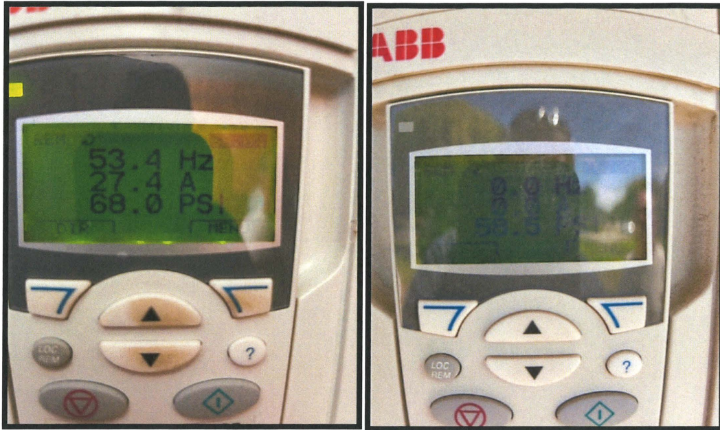
Photo 5 (Left) - VFD controller for Well #1 pump running. Photo 6 (Right) - VFD Controller for Well #2, the pump operates under increased system demand.
