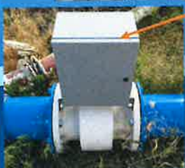
Protected meter head, this is probably the best that we have seen in the field.
