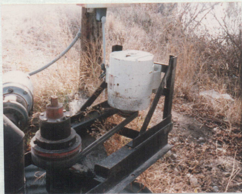
Pump A Parma Water Lifter with General Electric 7.5 h.p.
