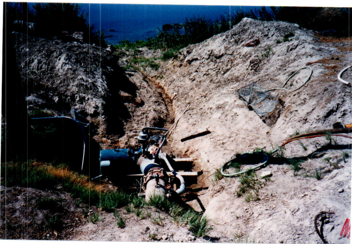
Snake River in the background. Pipeline from river to a CMP sump.
