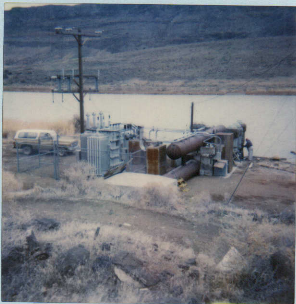
The pump station for Sinker Butte Canal
