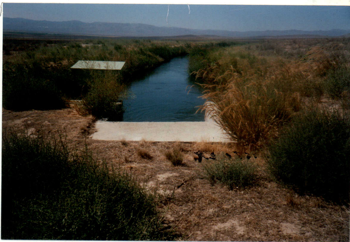
outlet of penstock - canal furnishes water
