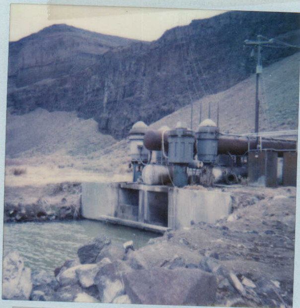
Sinker Butte Canal pumps
