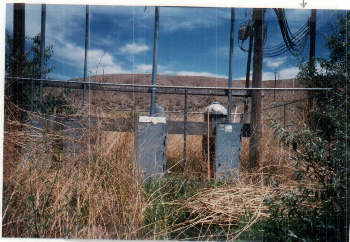
Reservoir Pump Station Looking East
