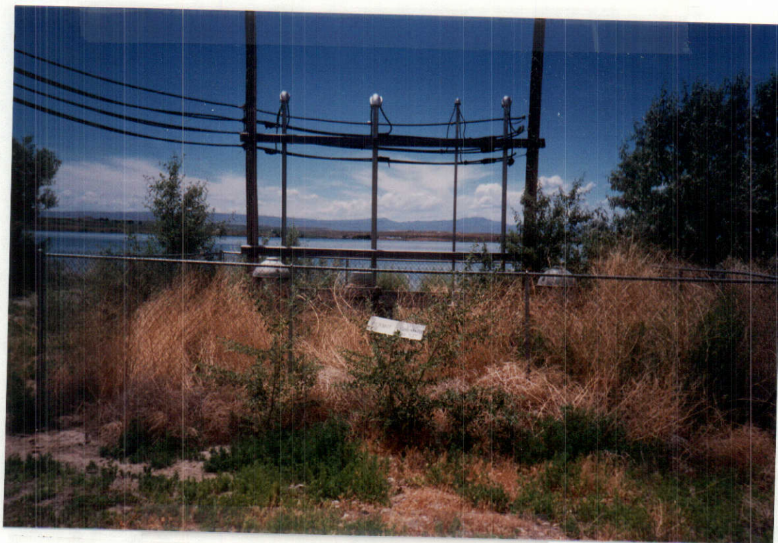
Reservoir Pump Station Looking West
