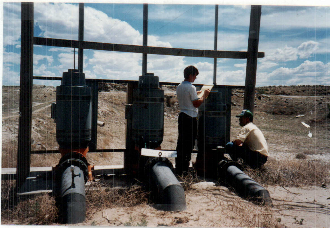
Hardina Pond Booster Pumps View Looking South.
