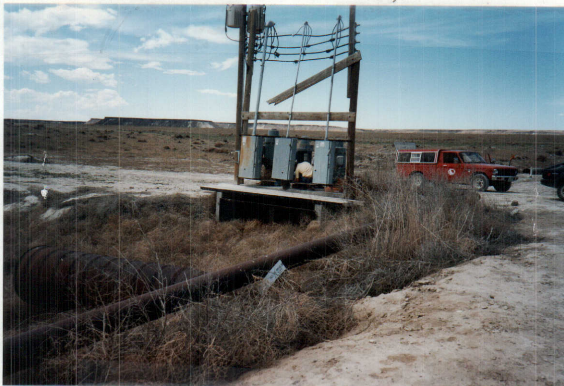
Booster Pumps AT END of ENLARGED DITCH. View Looking North West
