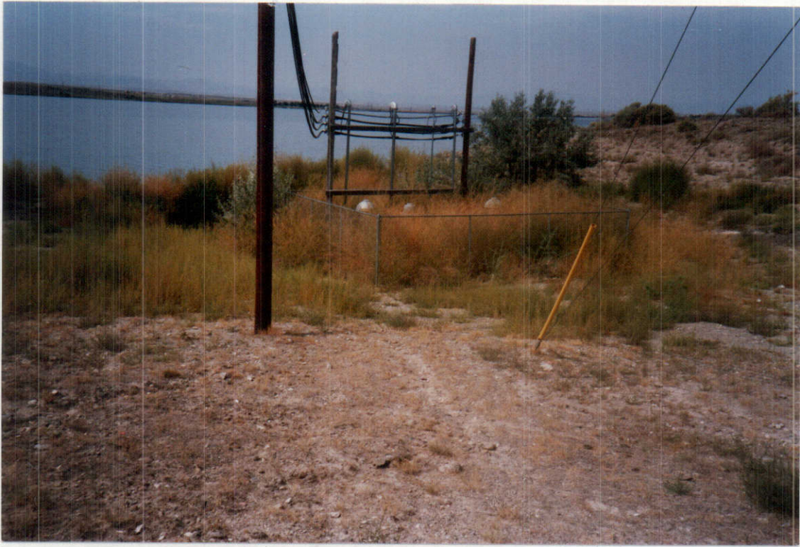
J.C. Strike Res. in the background. 4 pumps in the fenced area. 2-150 HP 1-100 HP 1-200 HP. NOT used in 1987.
