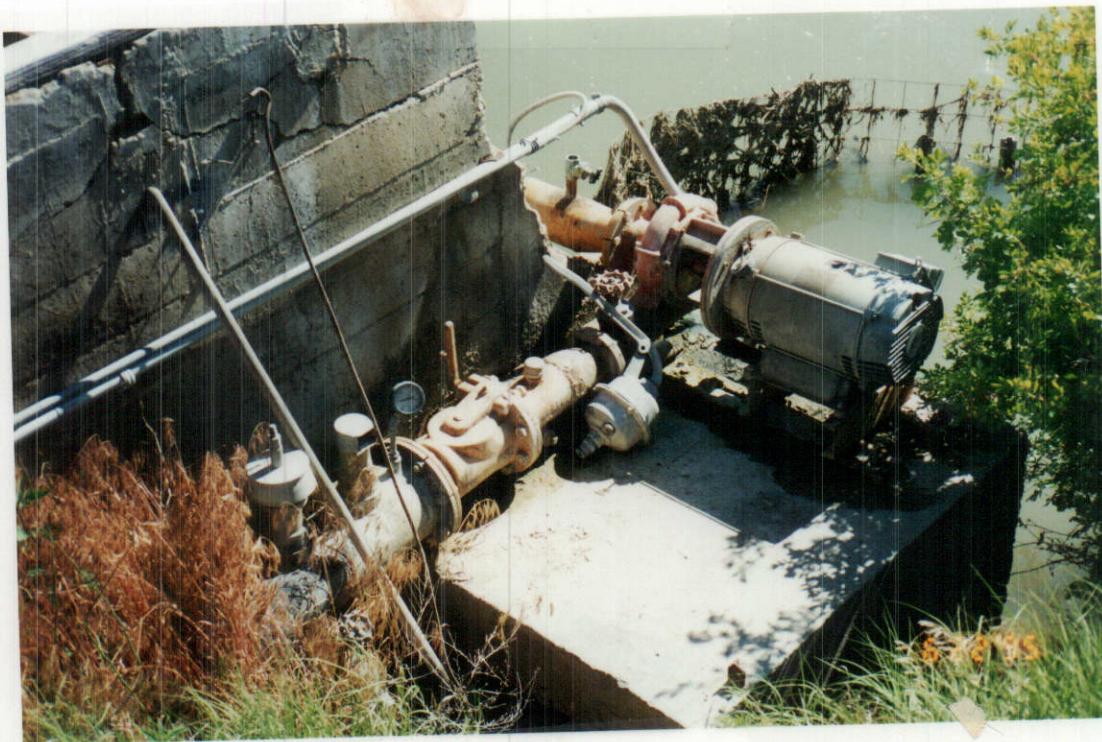
Sprinkler pump 40HP
