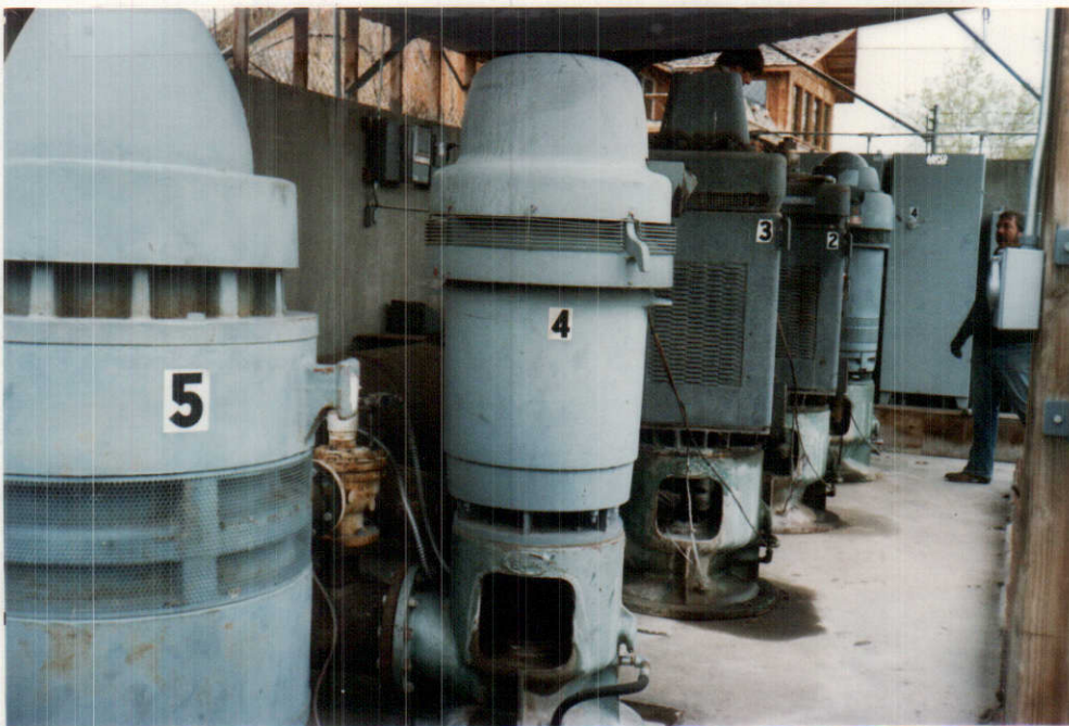
Interior view of Pumping Plant.
