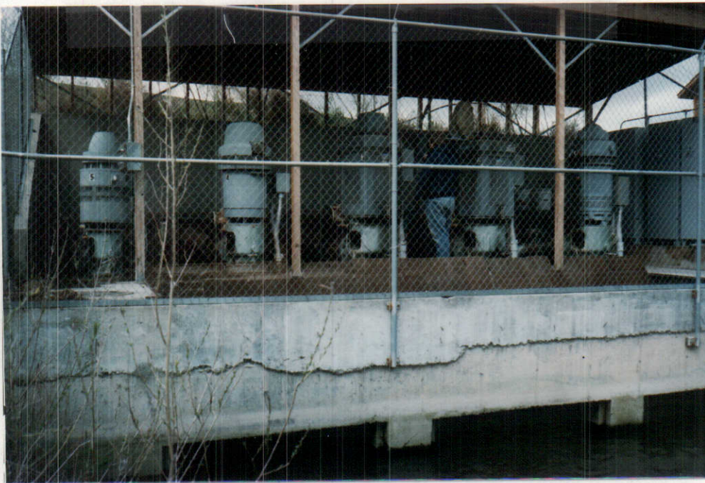
River intake & Pumping Plant
