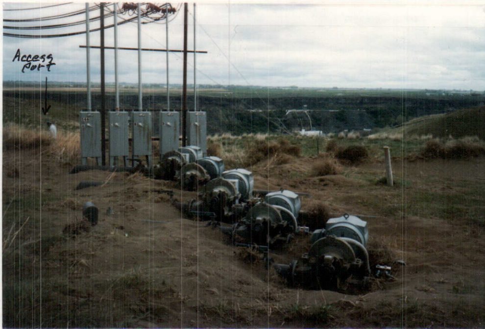
850 HP Booster Plant
