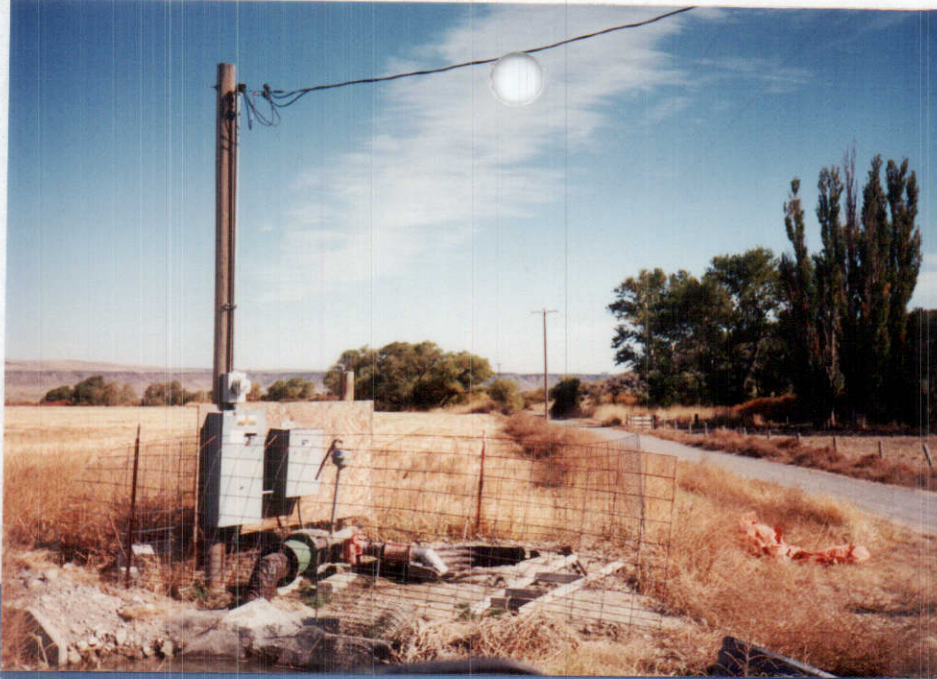
West Relift Station SESW S34
