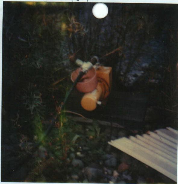
Electric Pump used to pump water from South fork Clearwater R. for irrigation L. L. Lee
