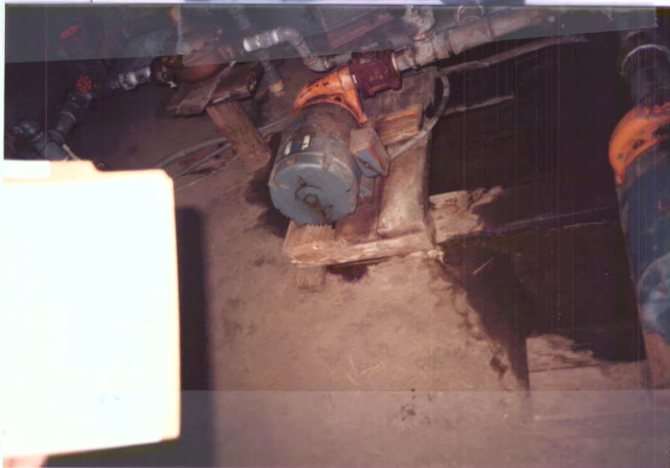
THESE TWO WELLS DELIVER WATER TO THIS STORAGE RESERVOIR SHOWING TWO 5 HP PUMPS DELIVER WATER TO 6" PRESSURE MAINLINE
