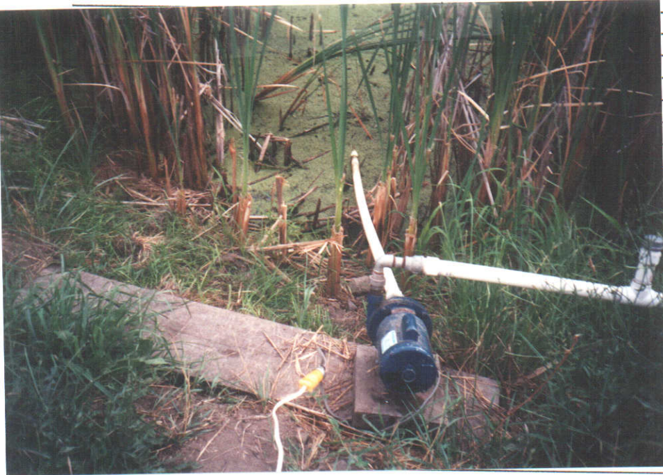
#1 pump in pond
