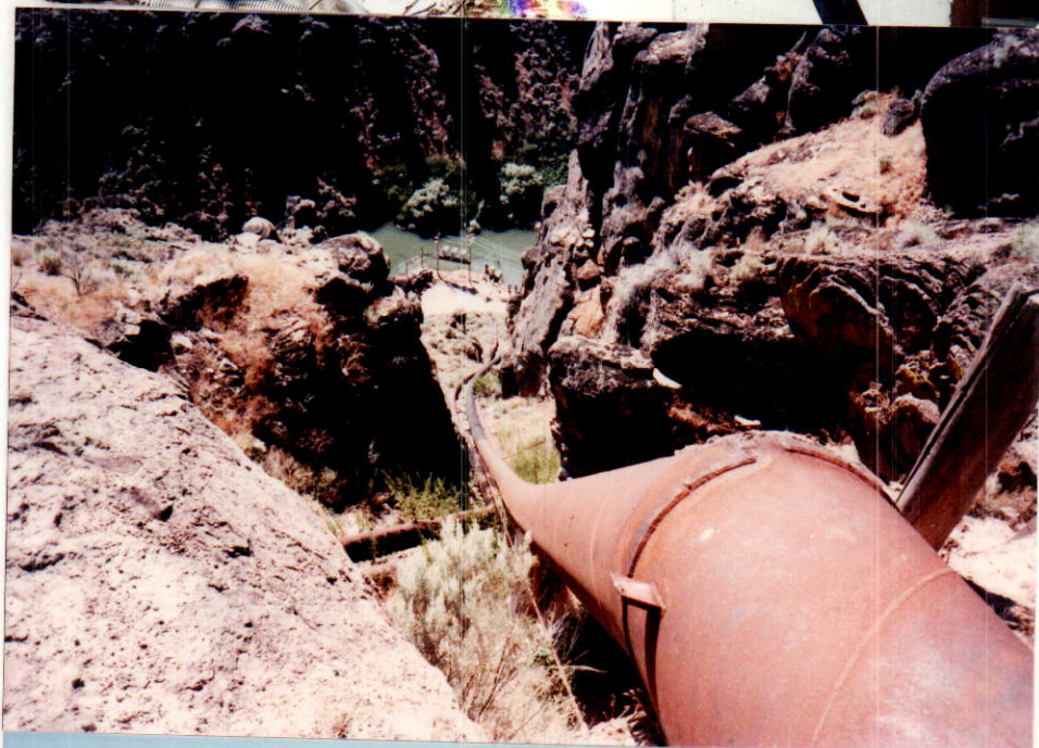
Pipeline from pumps to ditch.
