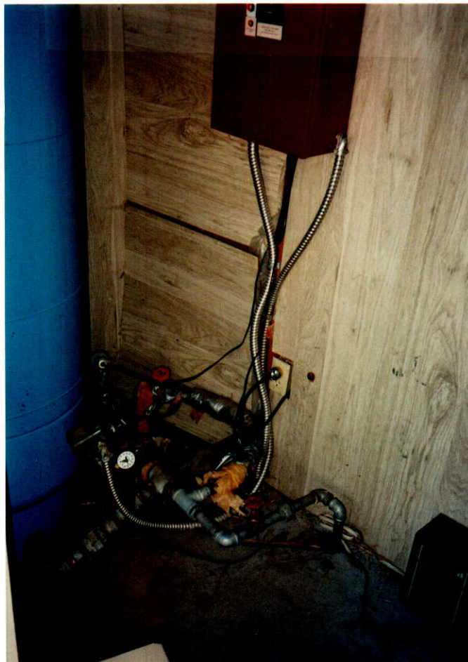
pipng, tank for well ①
