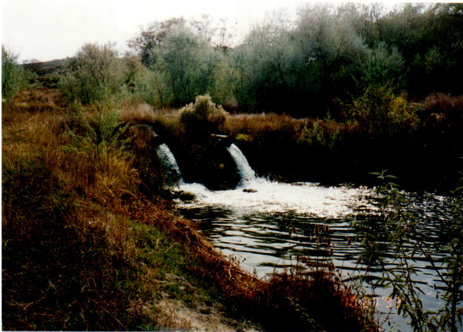
#4. Two 18" steel pipe that deliver water from ditch to Fish pond
