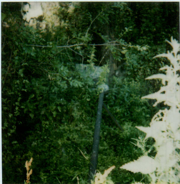
Pipelines From Springs
