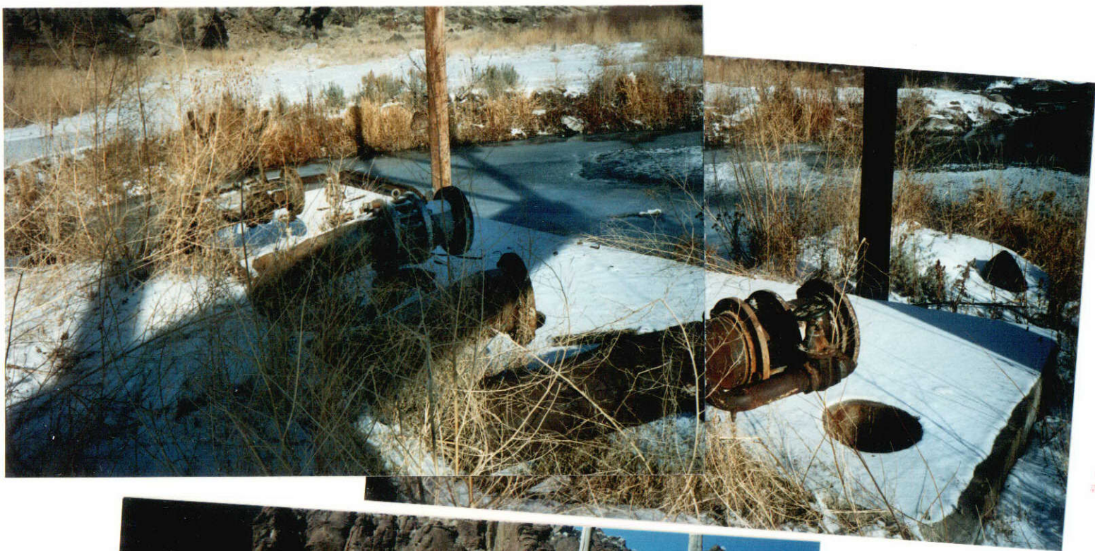
Lower Pumping station's
