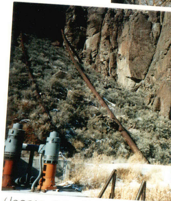
Upper pumping stations
