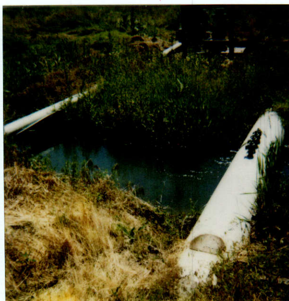
Mainline From Re-lift Pumps Across Feeder Ditch
