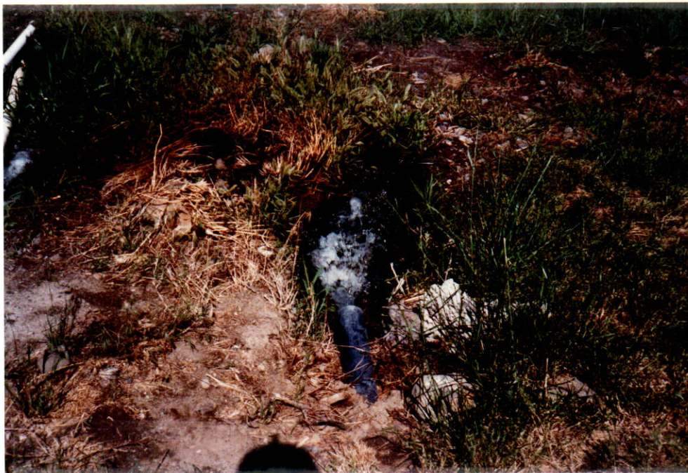
Hot tub effluent into ditch
