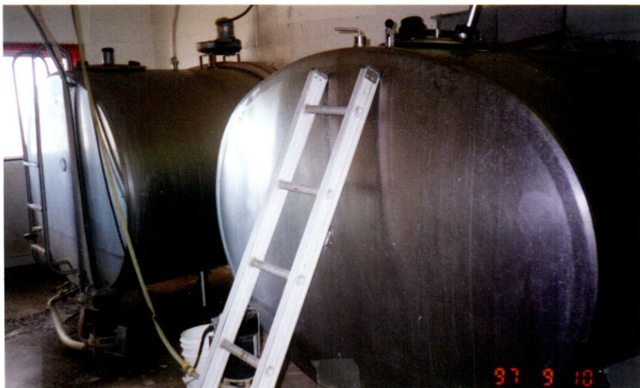
View of bulk tanks in dairy barn. The smaller of the two bulk tanks holds 2,500 gallons. Refrigerant (instead of water) is used to cool milk.
