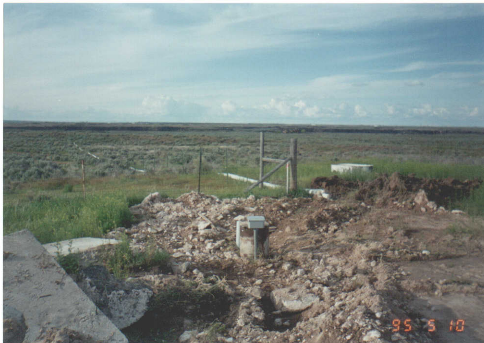
Figure 2 Stutzman 47-08019 Well with Submersible Pump
