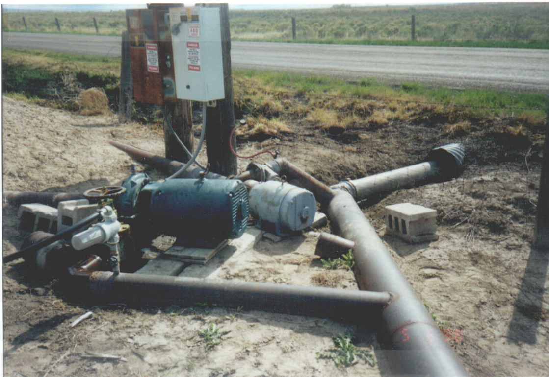
Re-lift Pumps N of Pond (Looking SW)
