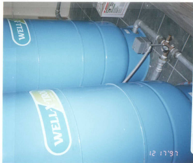
2 pressure tanks, in the pump house 45 PSI @ gage
