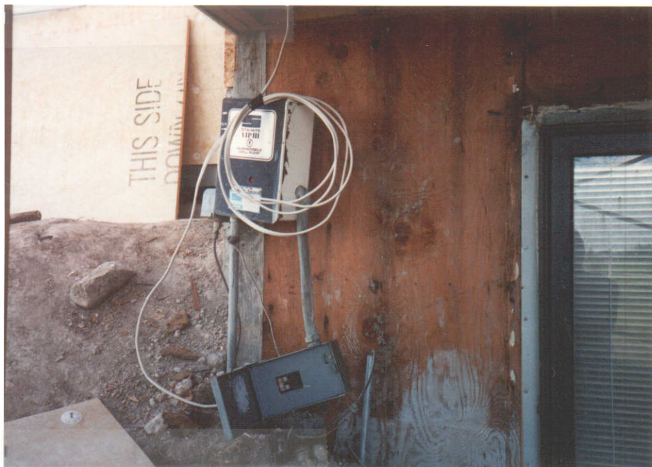
control box for PD ②
