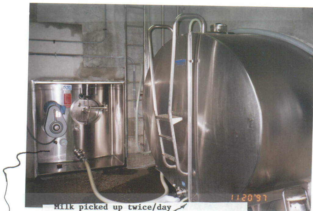
Pro-Chiller aka Heat Exchanger
