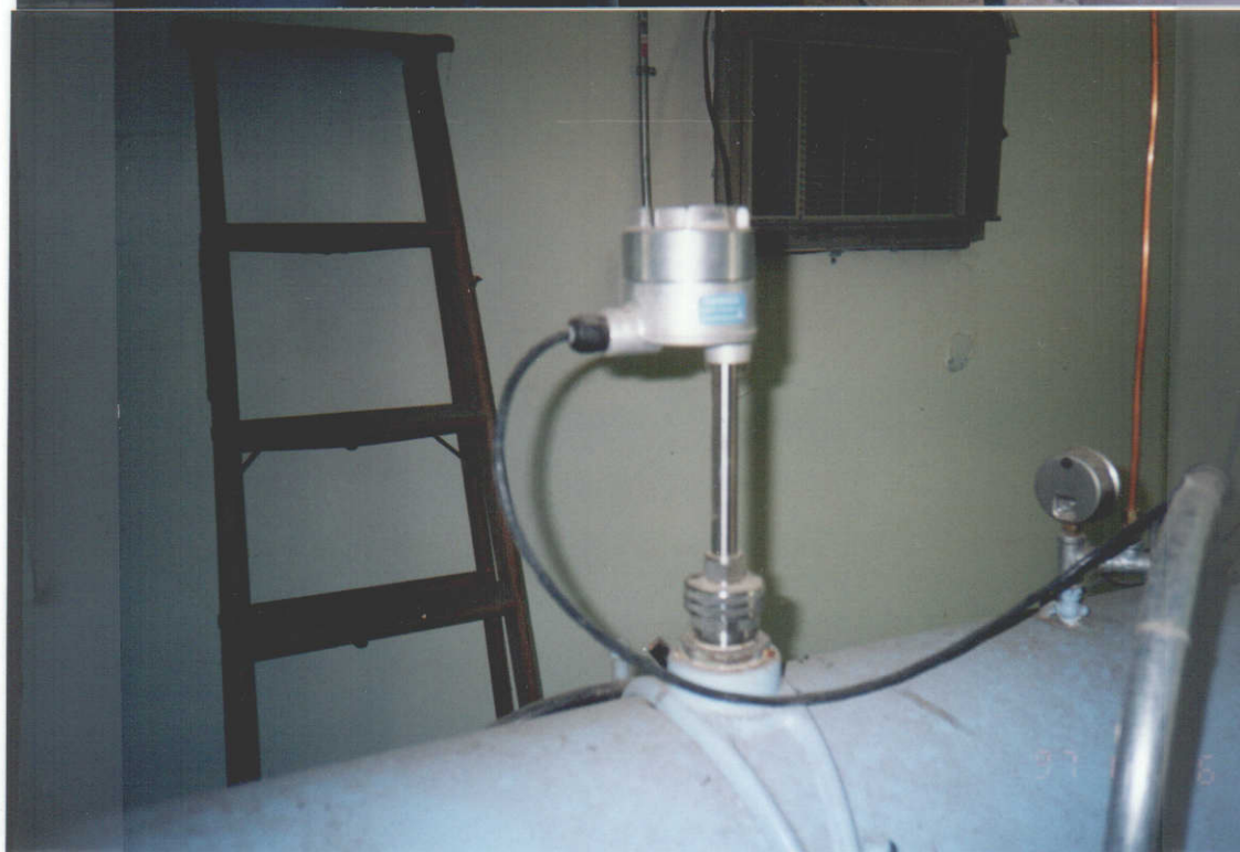
Buhl Well #5 & Flow Meter
