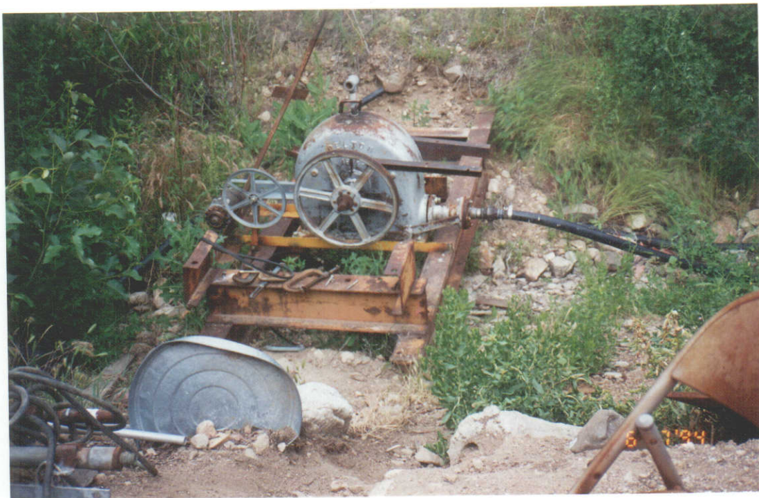
P/a Pelton wheel for power generation
