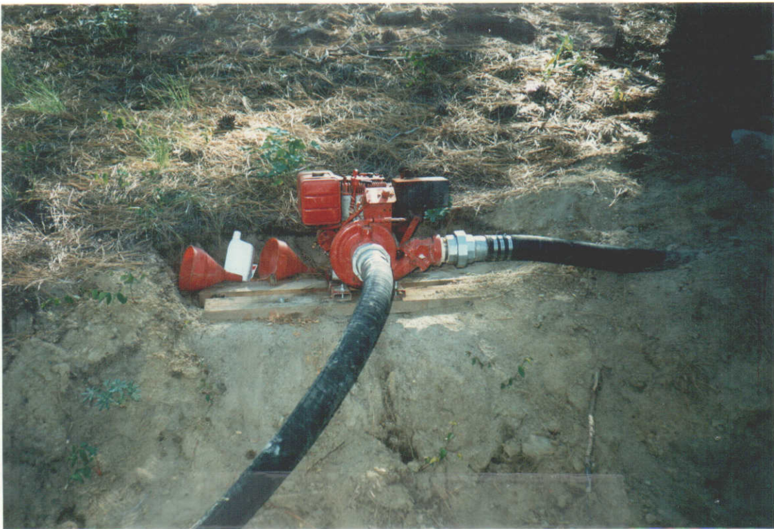
11 HP GASOLINE BOOSTER PUMP
