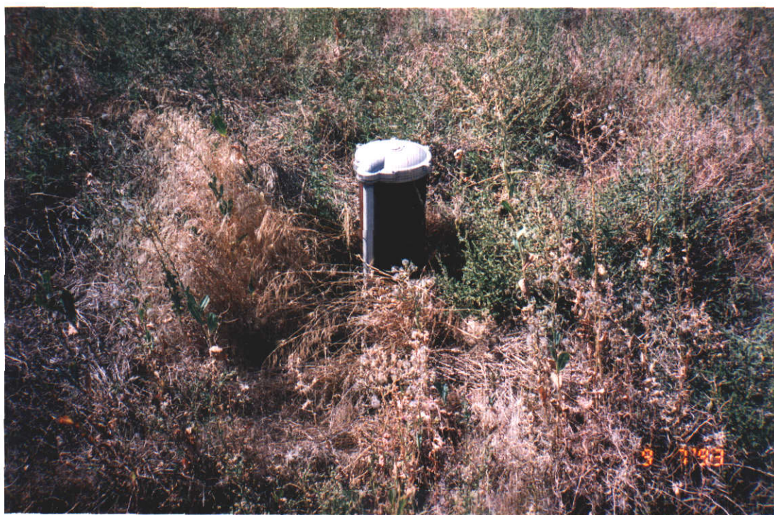
8" well 5 HP submersible pump
