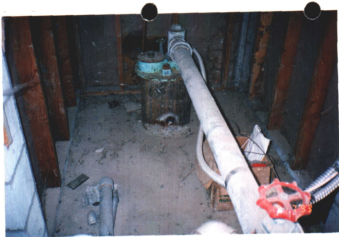
12" well 15 HP submersible pump
