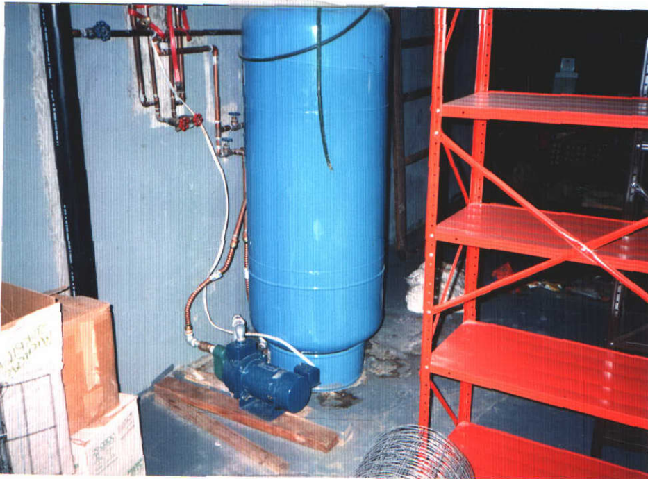
#4. Pump and pressure tank located in the basement of residence that services domestic internal use.
