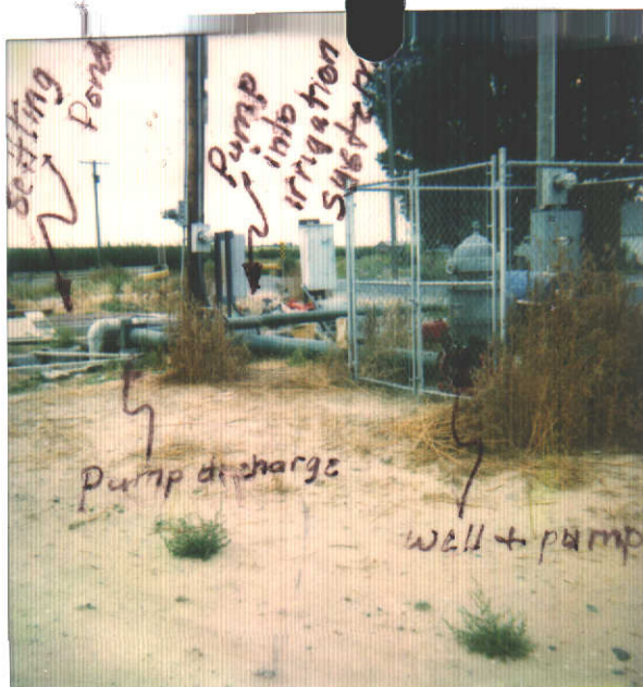
Looking westerly at the 2 pumps, and settling pond
