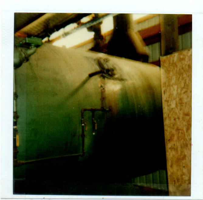
MINT STILL BOILER
