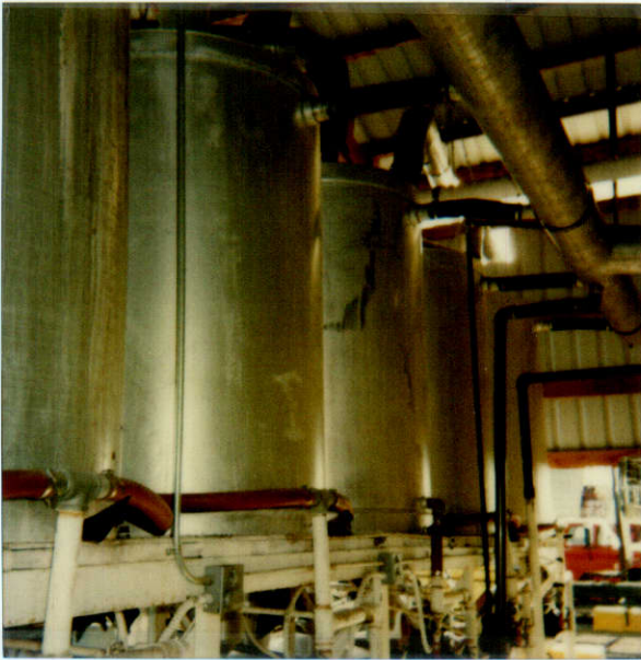
STEAM TANKS FOR STILL
