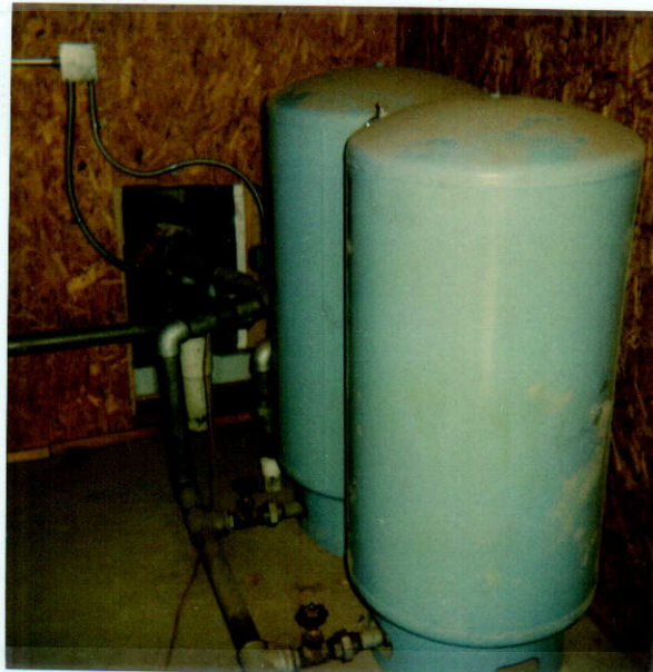
WELL AND PRESSURE TANKS
