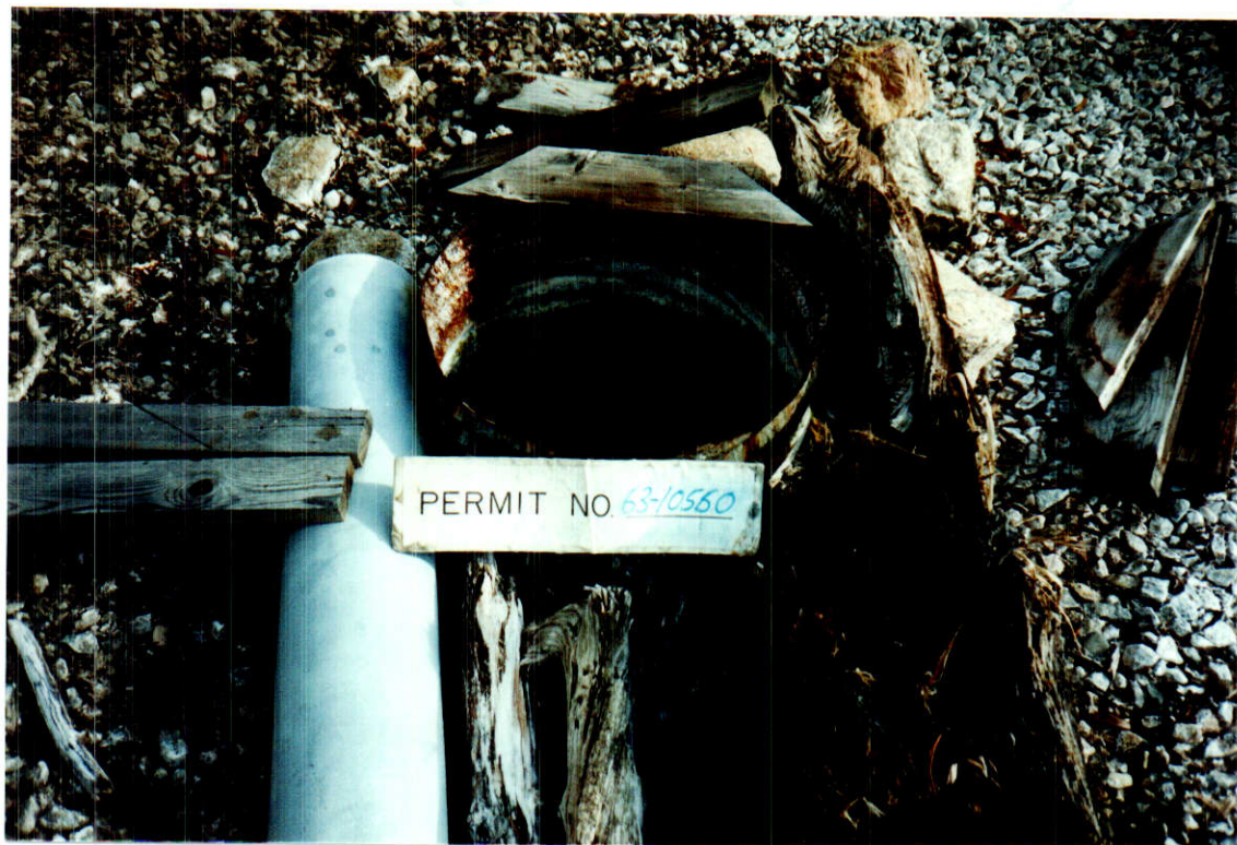
PHOTO THREE- Spring #1, PID is #1, is 63-10560. Collecting culvert has 3 lines to pump house in photo #4.
