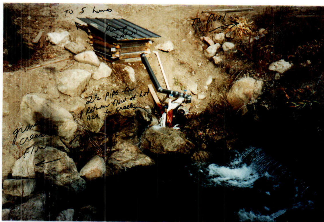
PHOTO TEN- Pump station #2 provides hot water to 5 homes at NE end of subdivision. 16" line from pool ends at pump station. Return H 2 O from 5 homes discharged to creek via 2 1/2" pipe (used 5 gallon bucket measurement on return flow). Gross ck. shown in foreground.
