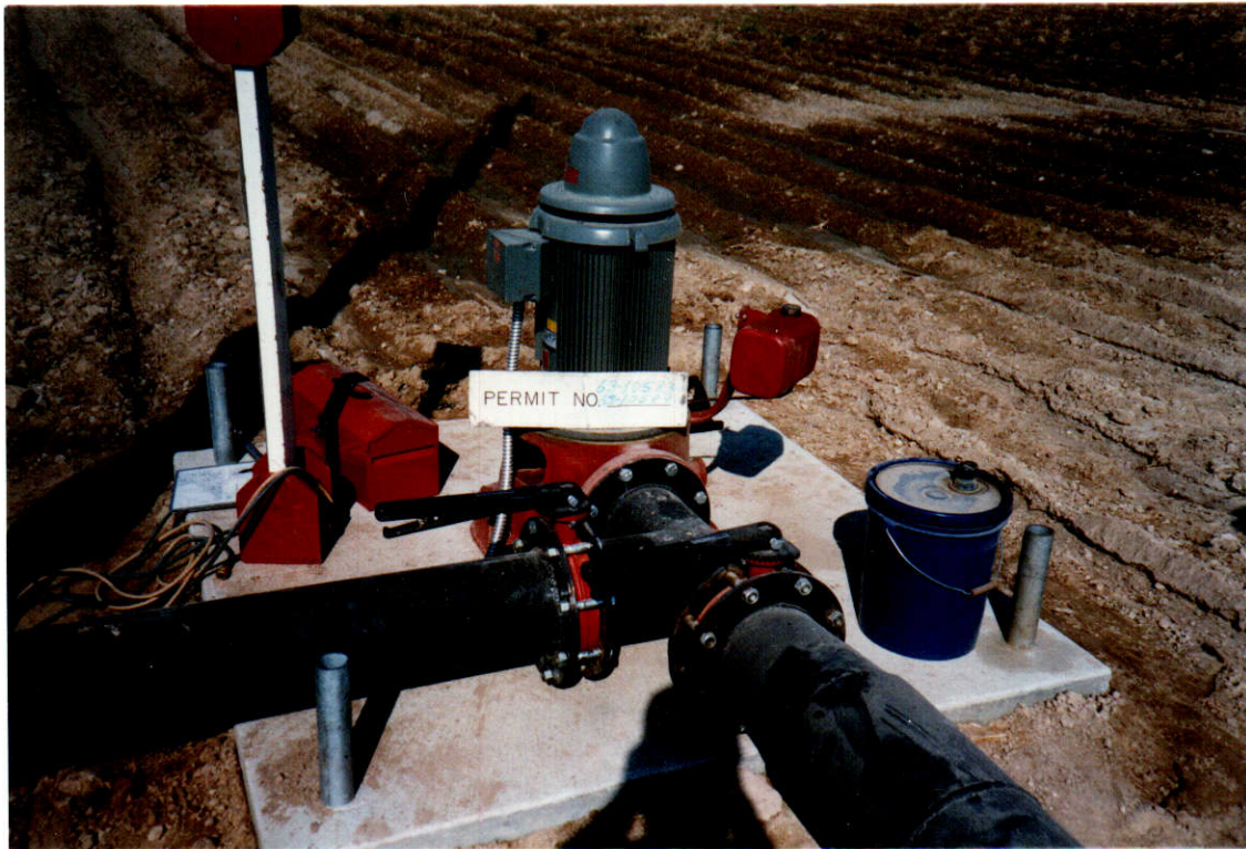
PHOTO ONE- Point of diversion for this right and 63-10584. Access port is just out of view to left.
