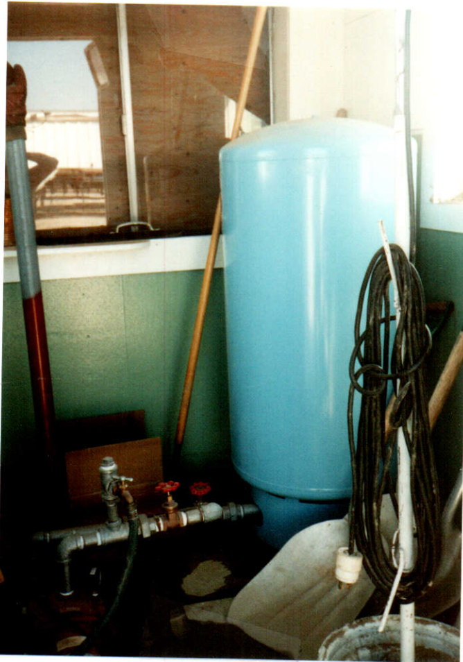
#2 Pressure tank located inside well house.
