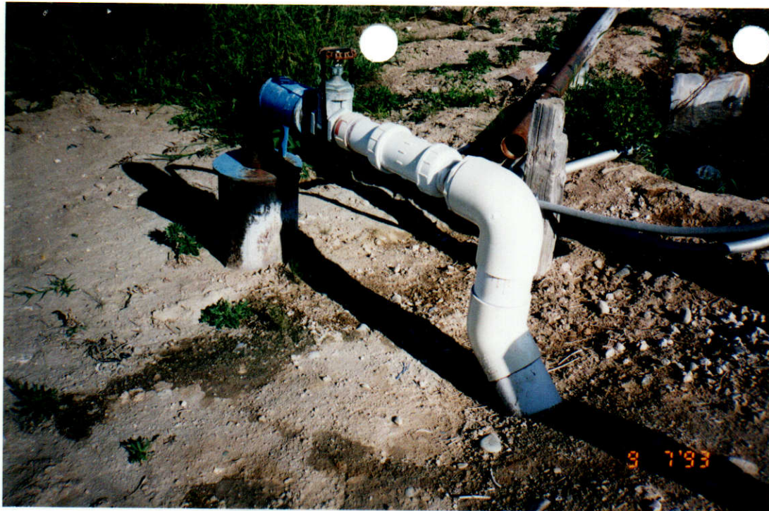
12" well 25 HP submersible pump
