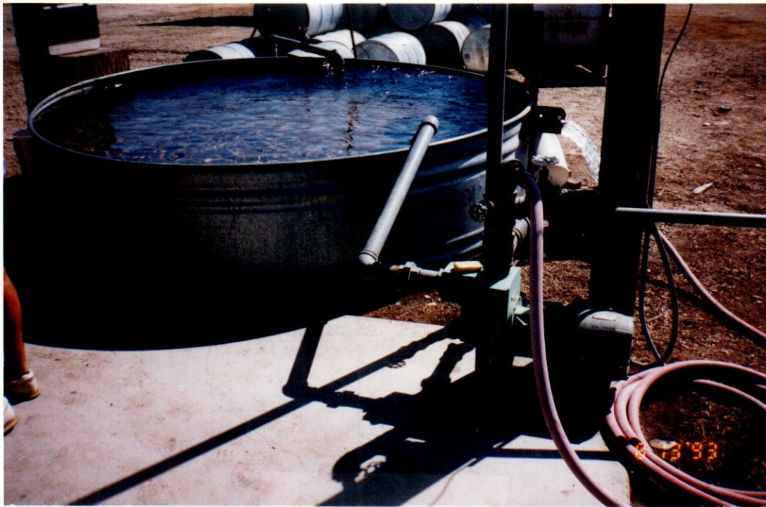
5 HP Booster pump
