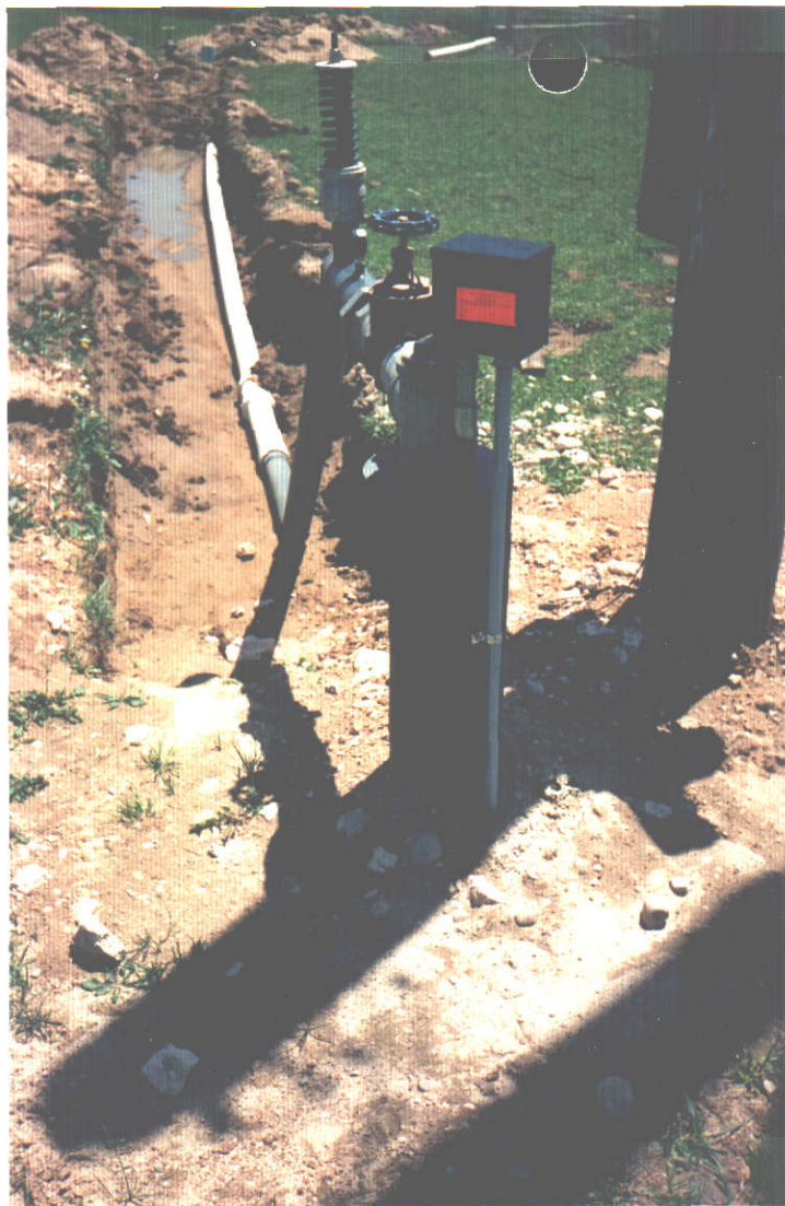
8" well 10 HP submersible
