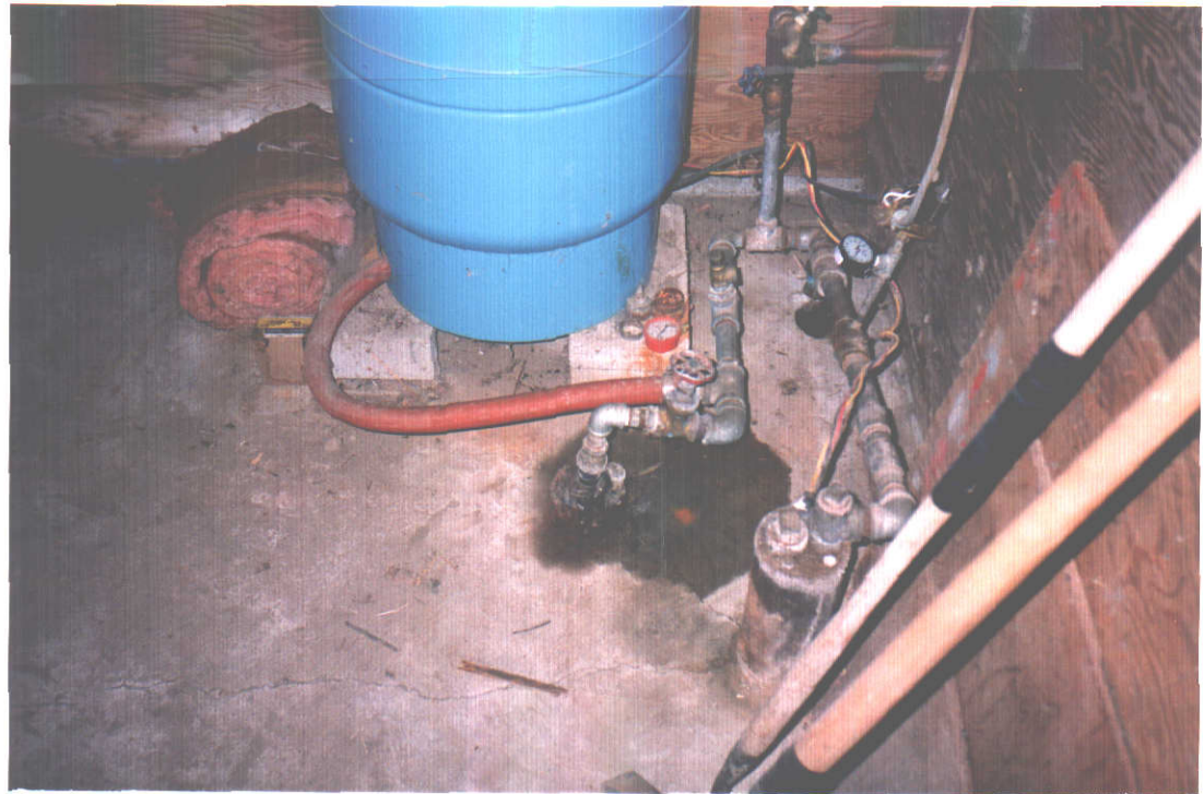
PHOTO ONE- Well, 4" casing, and pressure tank in well house.
